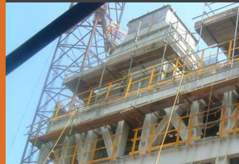
Traditional WHRU: 70 tonne. Support structure: 100 tonne (3 units)
